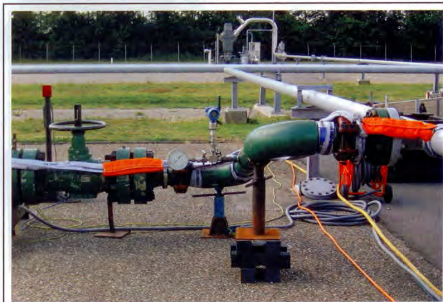
Nederlandse Aardolie Maatschappij B.V. is using wireless sensors to measure differential pressure and temperature as part of a mobile wellhead test system. Wireless systems are enabling companies to automate more processes.
